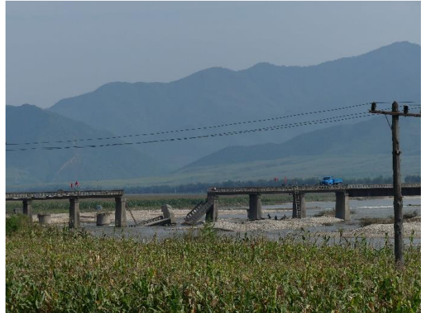
Photo 14: Damage of bridge by the flood.
