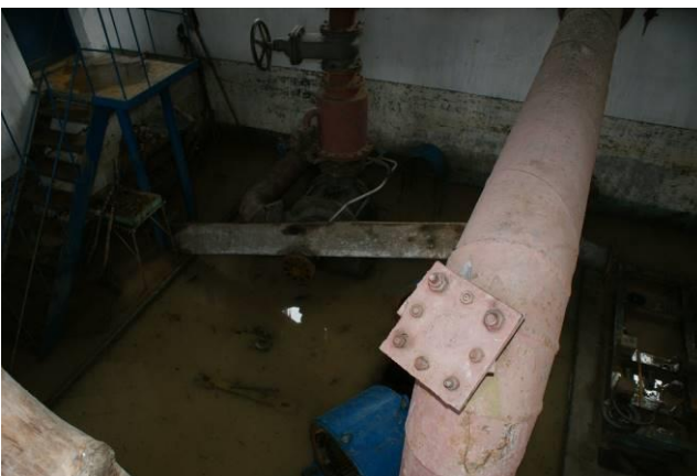
Photo 17: Flooded and destroyed pump house which supplies water to Hoeryong city centre.
